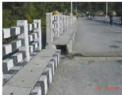
E-W shift observed in the span of Panighat bridge near Diglipur
