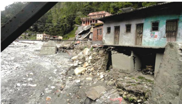
Figure 5. Highly damaged flood protection wall on the left bank of the Asi Ganga near the confluence of the Asi Ganga and Bhagirathi river at Gangori township.
