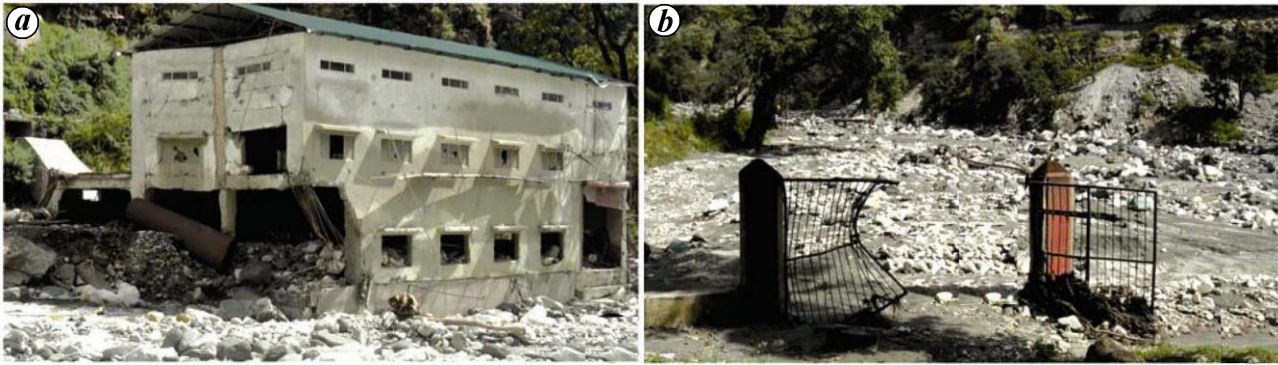
Figure 4. a , Highly damaged power house located near Kaldya in the tributary Asi Ganga. b , Remains of school entrance at village Kaldya that has been completely washed away.
